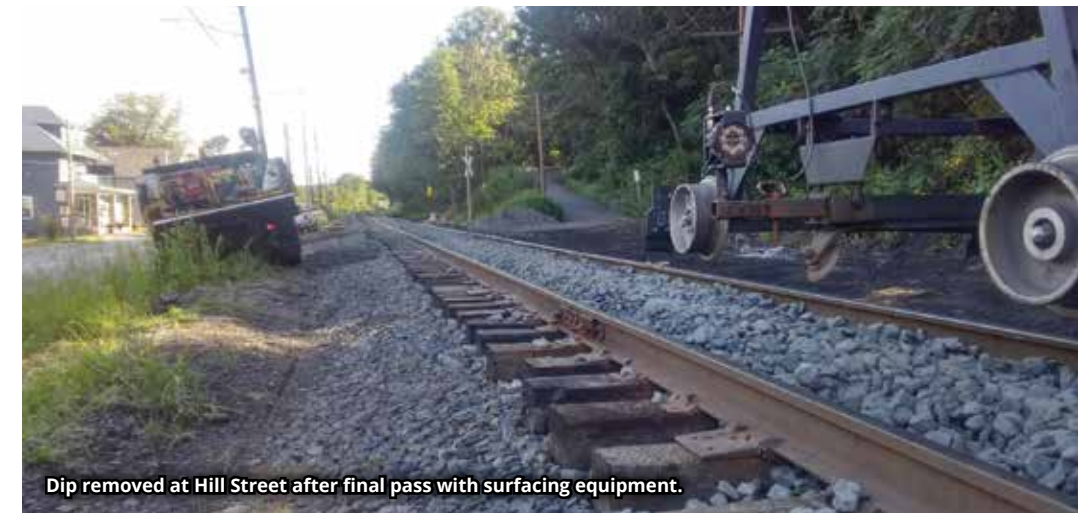
Complete crossing removal at Moosic Rd. Scranton Branch MP 3.39 D Zimmerman in PT-1, A. Scubelek in backhoe.
