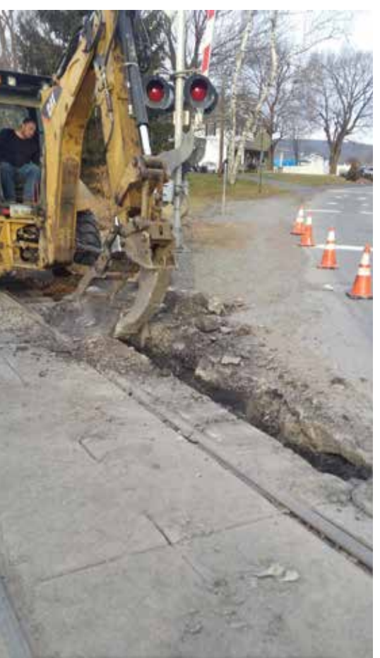
Operator Alex Scubelek Jr. removing asphalt in preparation for a complete crossing rehab.
