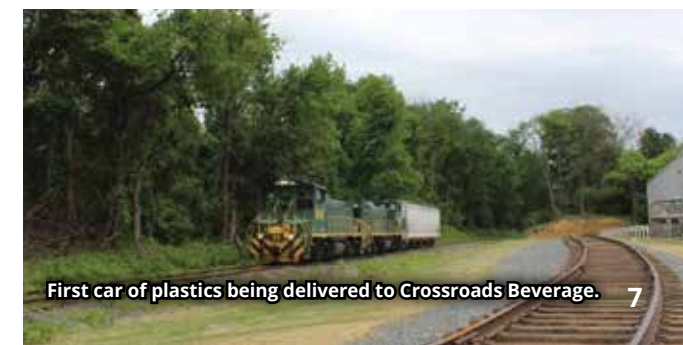
Rail unloading system with new rail siding is almost done and ready for first cars.
