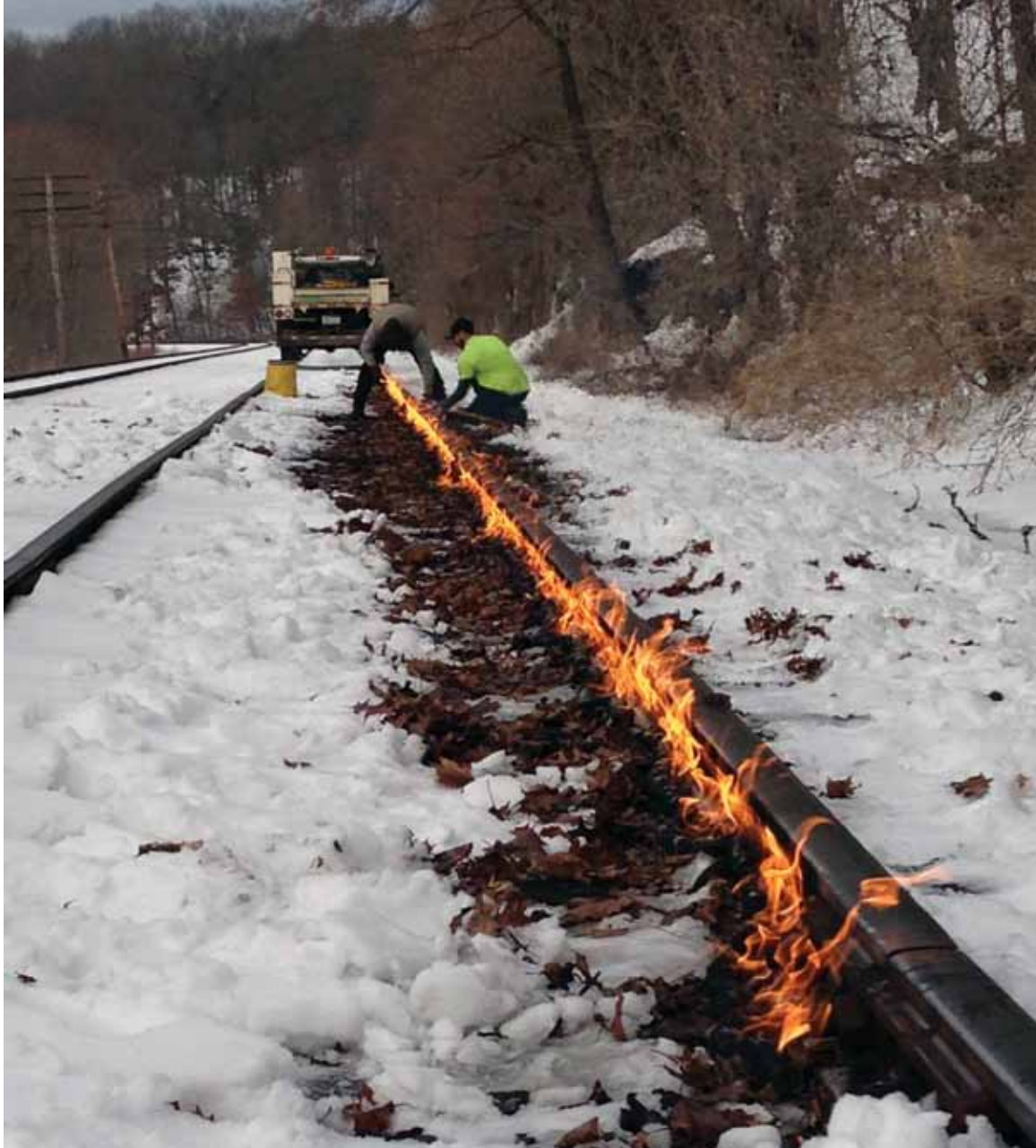
Frank Sebelin and Matt Minnich repairing a pull apart on the Lehighton branch.
