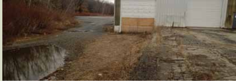
"Before" photos of track leading into the warehouse covered with dirt.
