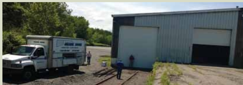
Rebuilt track and new rail car door providing increased clearance for modern hi roof boxcars.
