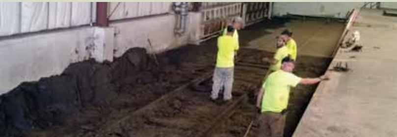
Track crew has removed dirt covering the track inside the warehouse in preparation to replace ties and ballast.
