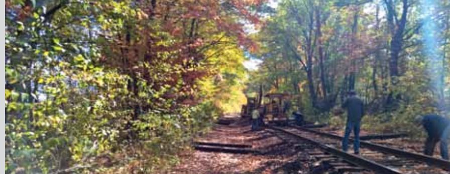
W. E. Yoder tie installation gang in full swing to install ties north of Tamanend Road Crossing MP 1.24. Andy Muller stands just right of center of photo on the track inspecting the work.
