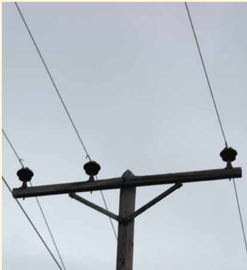
What a line looks like without the device installed.
