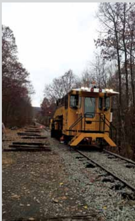
The Mark IV tamper hard at work finishing the work area after ties have been installed, ballast dumped, and a 3 inch raise applied to the track north of Mauch Chunk Junction MP 0.63.
