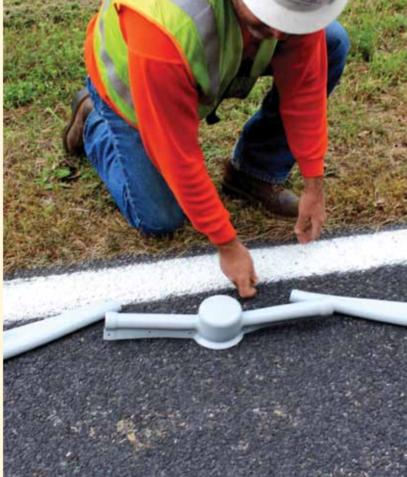
A close up of the rubber pieces that are being installed on the wires to prevent a circuit from going through a perched hawk.
