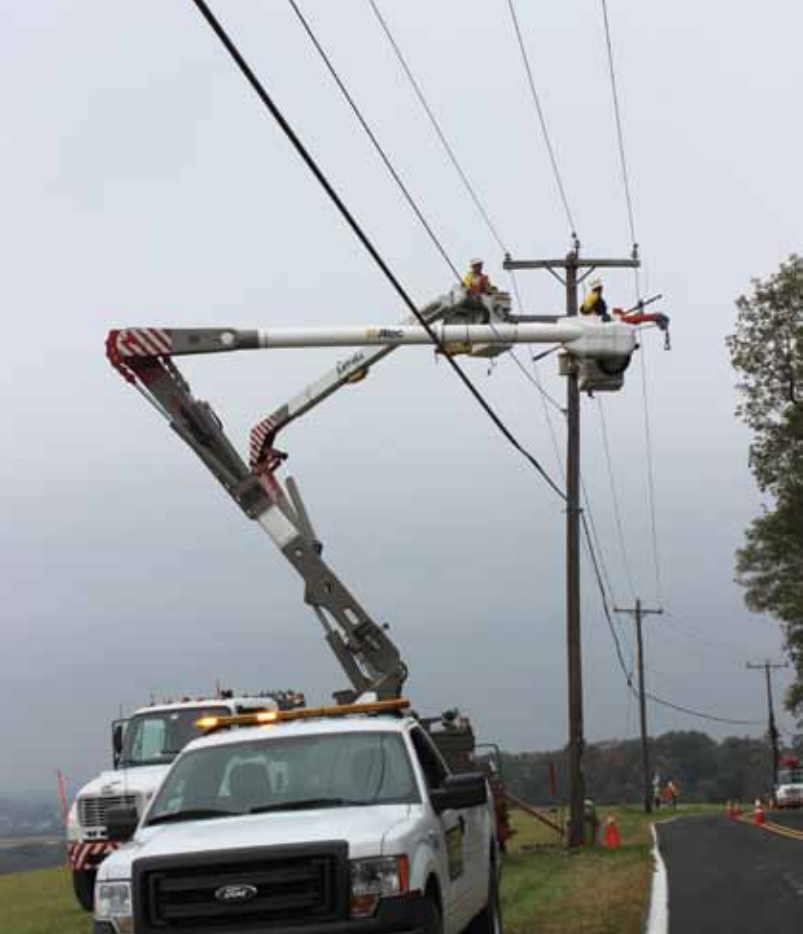
Met ED crews installing the protection devices on the wires where the hawks rest.
