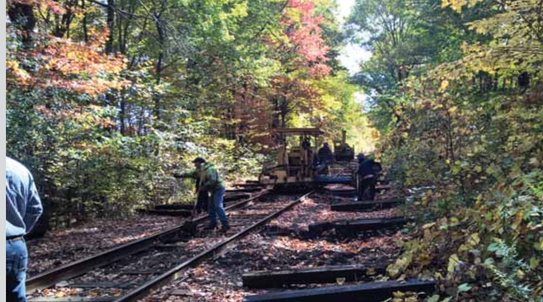
W. E. Yoder tie gang installing ties on Hazleton Line just south of Main Street Quakake MP 1.84. As the gang installs new ties, 18" double shoulder tie plates are also installed on each tie.
