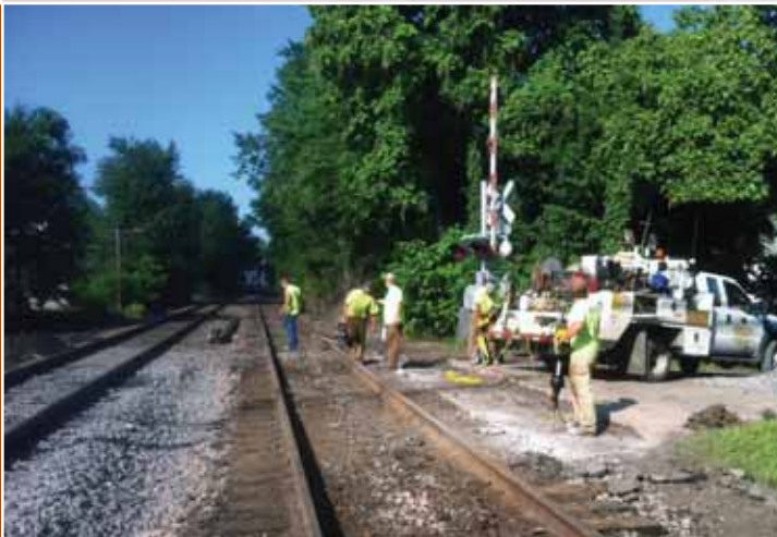
Looking south at Main Street MP 175.19, #1 track is finished begin surfaced as MoW forces begin again on #2 track crossing. Double crossings are twice the fun! As soon as one is done, another one awaits.
