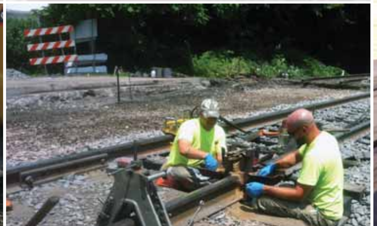
Setting up thermite welding on one of the Main Street MP 175.19 crossings. It is a very meticulous process that leads to a good weld. Shortcuts can lead to failed welds and more work.
