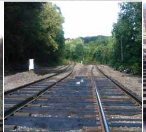
All new switch timbers installed for the two new #20 switches at Dupont MP 175.5. This view is looking north to the CP connecting track and the Susquehanna branch.
