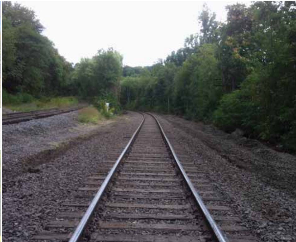
Standing on the Susquehanna branch with the CP connecting track to the left, the track will be realigned to accommodate a #20 equilateral switch making both #1 track and #2 track accessible at the beginning of the Susquehanna branch at Dupont MP 175.5
