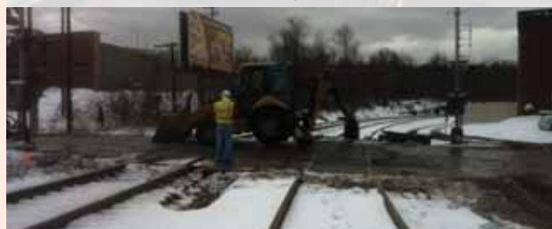
With a full road closure begun at Oak Street MP 173.13, the backhoe starts removal of all the old materials on #2 track.
