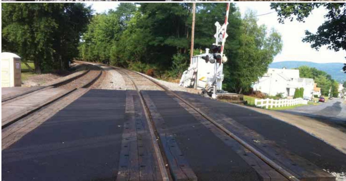
Looking south on #2 track at Broad Street MP 174.56 after it received a much needed facelift.
