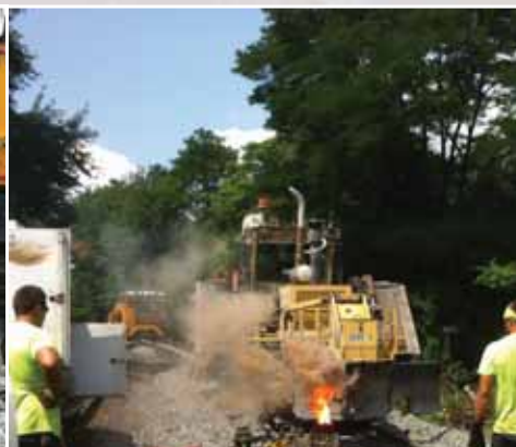
Thermite welding new rail in the #2 track Broad Street Crossing at MP 174.56. A little volcano adds some heat to an already warm day. Left to Right: Matt Nester, Matt Minnich, and Larry Weller.
