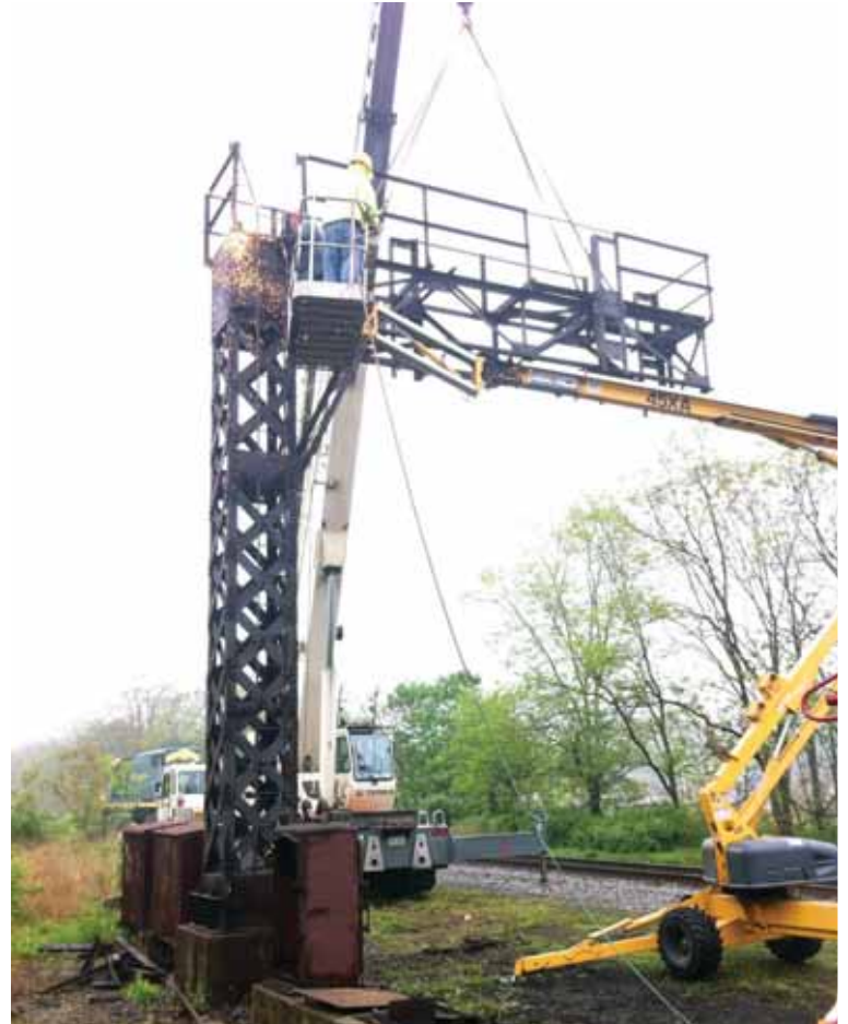
With assistance of Tom Day and John Walaitis, cantilever begins to be taken apart.
