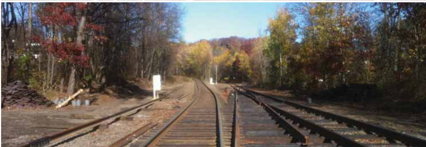
Halfway through the realignment of the new tracks, CP connecting track and the Susquehanna branch, the equilateral switches are installed and being finished at Dupont MP 175.5. A few more steps in constructing the switches and we will be ready for surfacing!
