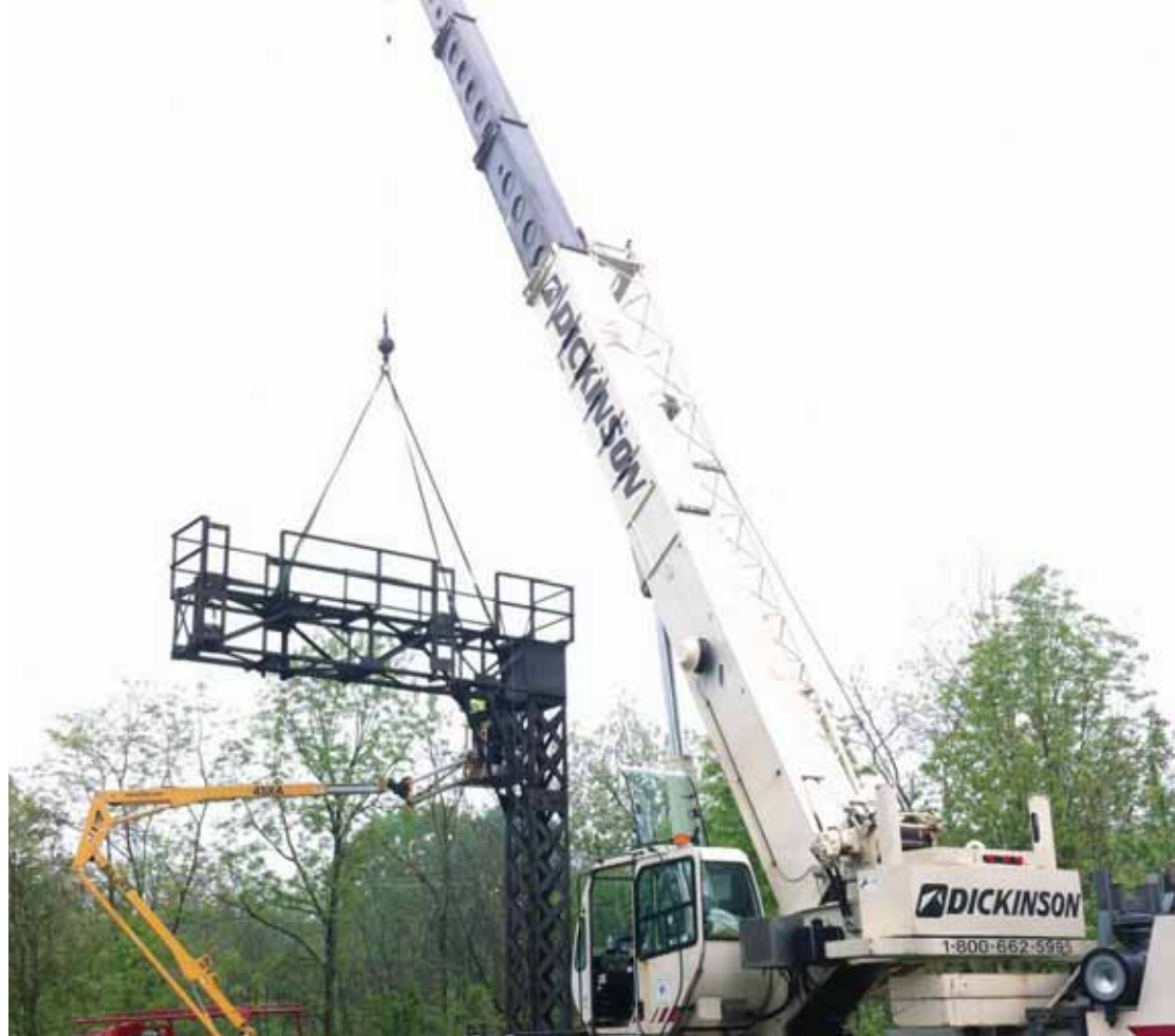
With the help of Dickinson Crane, cantilever will be disassembled and transported to Port Clinton on a flat car for cleaning and modification.
