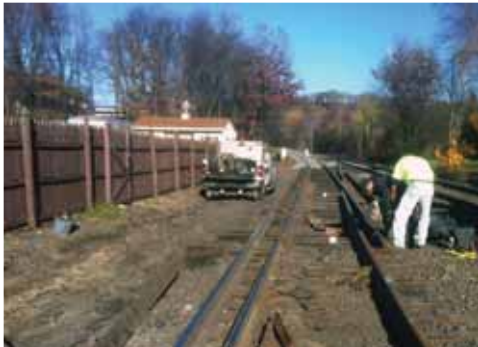
In the far distance, the two new #20 switches are installed. Fresh ballast has been dumped and the MoW forces now focus on rehabilitating the two #15 switches at Dupont MP 175.5.
