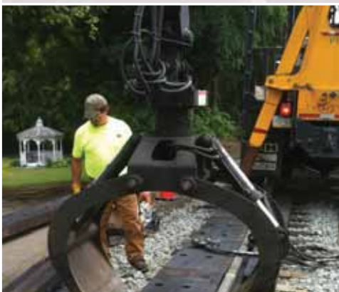
Last step in rehabilitating #2 track crossing is installation of the crossing timbers so the new asphalt can be laid out at MP 175.56 Broad Street. Left to right: Vince McGuigan and Aaron Cassel.
