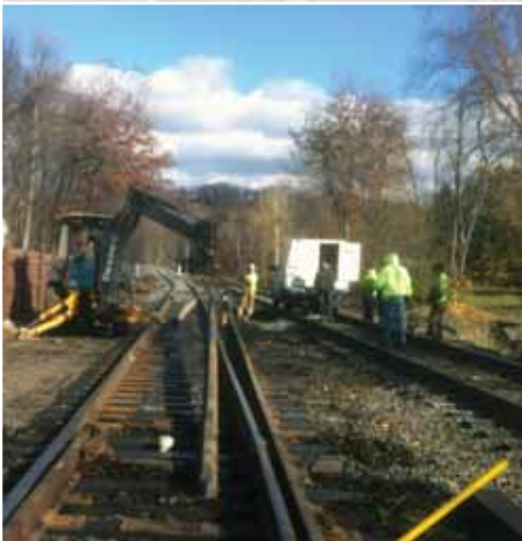
MOW forces are busy constructing a #20 equilateral switch at Dupont MP 175.5. The closure rail is being set into place by the backhoe as the switch continues to become part of the new interlocking.
