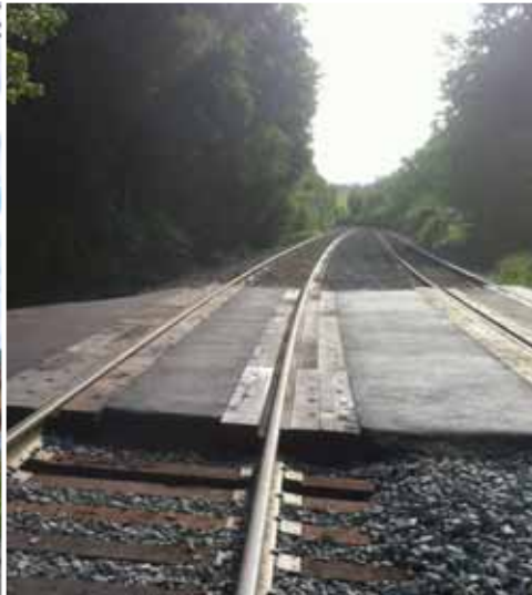
Newly rehabilitated #2 track crossing at Broad Street MP 174.56 after it received new ties, surfacing, crossing timbers, and asphalt.
