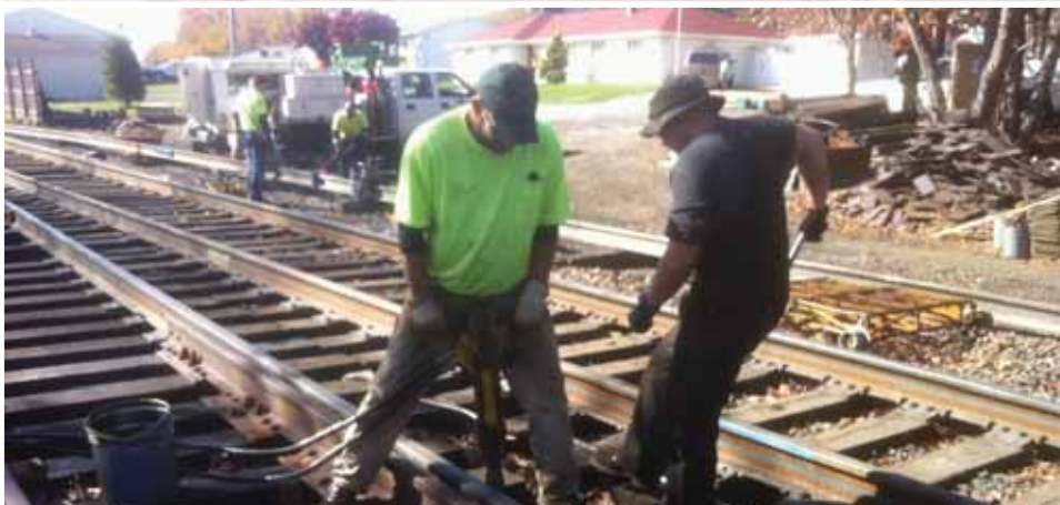
Adding some heat to close the gap as the finishing welds are added to the new #20 switch. MOW forces are standing on #1 track at Dupont MP 175.5 as the Signal can be seen behind the truck. The CP connecting track is to the right.
