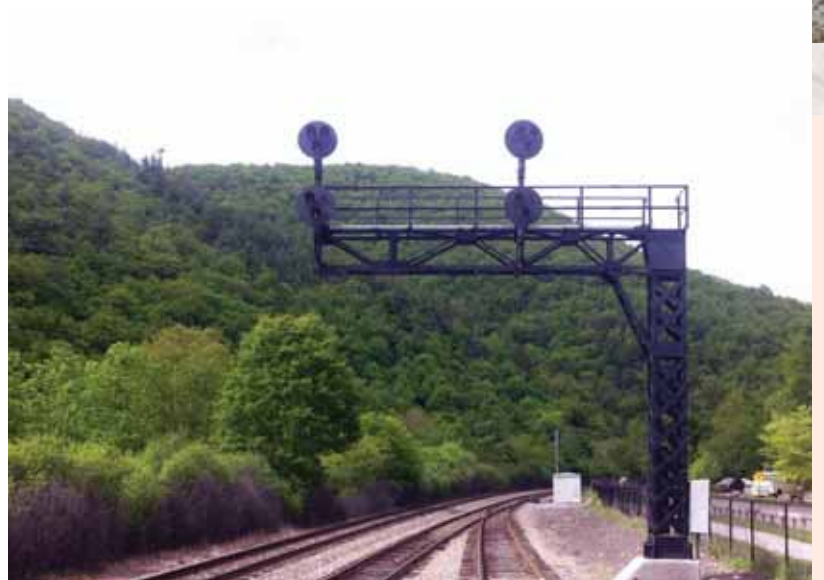
Completed interlocking in service.
