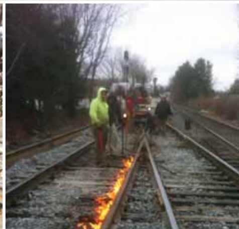
Installation of the guard rail on #1 track at Dupont MP 175.5. Spikes have been set and the hydraulic spiker is driving them down to finish the installation.
