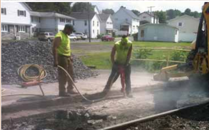
Some concrete was found under the road as MoW forces were rehabilitating Main Street MP 175.19 crossings. It was removed with little impact on getting the project done in the time allotted for the project.
