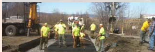
With a fresh base of ballast on #1 track at Oak Street MP 173.13, laying out new ties is in full swing. Many ties are marked, laid out and then matched to the correct tie spacing in the crossing. A vital step in matching the concrete panels to the ties.
