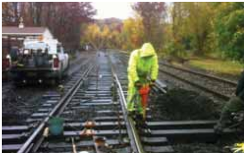
New switch machines are being added by the Signal Department on #2 track at Dupont MP 175.5 as MoW forces continue work on the CP connecting track in the distance.
