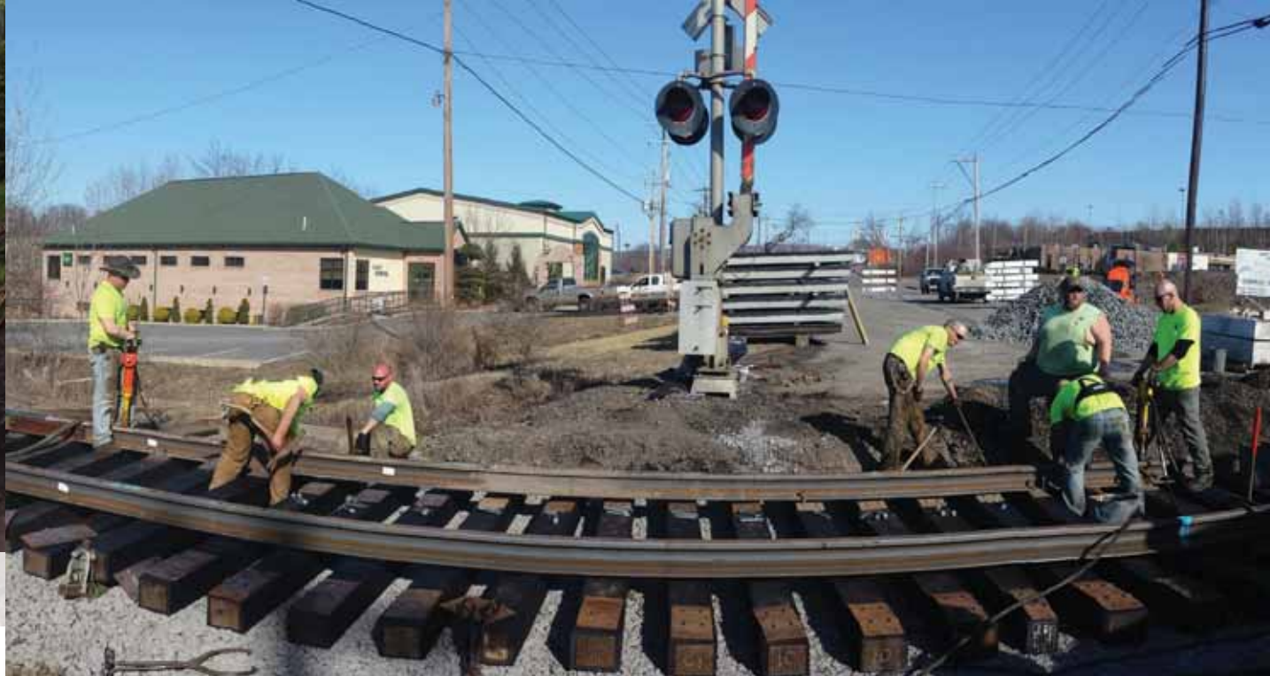
A panoramic view of the 45 foot long crossing on #1 track at Oak Street MP 173.13 as MoW forces are busy plating and spiking in the new rail onto the ten foot ties.
