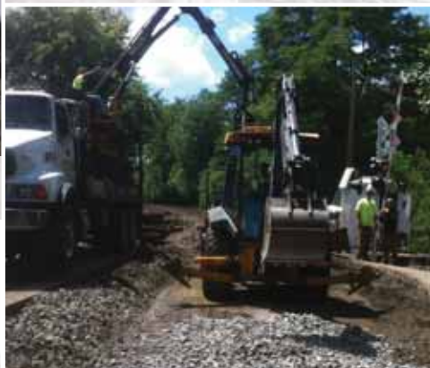
The old ties have been removed, new ballast is laid out, as the backhoe and PT-1 begin to layout new ties on #2 track crossing at Broad Street MP 174.56. Left to Right: Duane Zimmerman PT-1 Operator and Dale Homm, Backhoe Operator.
