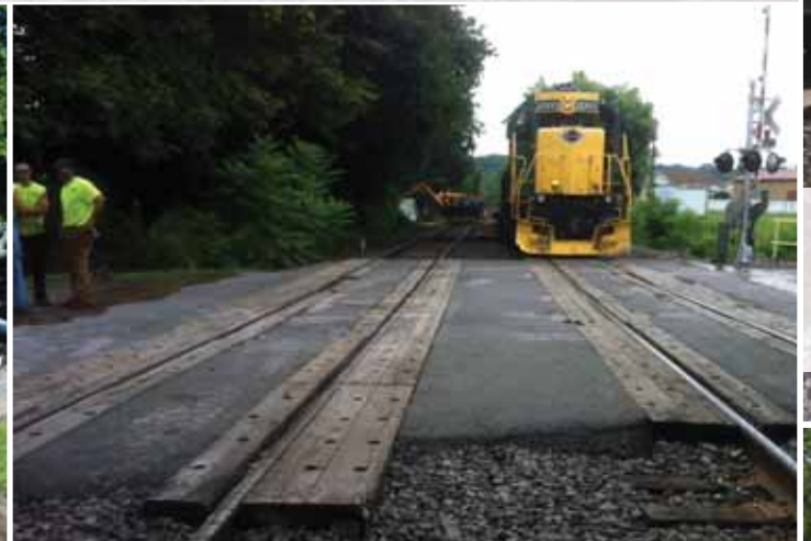
Main Street MP 175.19 crossings on #1 & 2 will soon be getting new concrete panels and surfacing for a new ride for both trains and vehicles.
