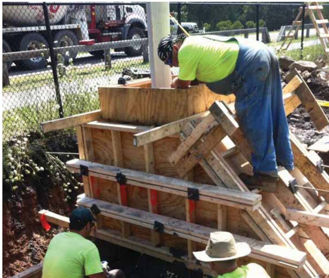
New foundation for Cantilever being poured. John Walaitis directing concrete as Mario and Dave assure no air voids are created.
