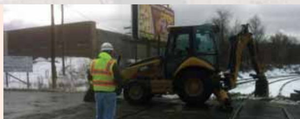
Oak street crossing replacement MP 173.13 began on a snowy day. This crossing had the rubber crossing mats replaced with concrete panels.
