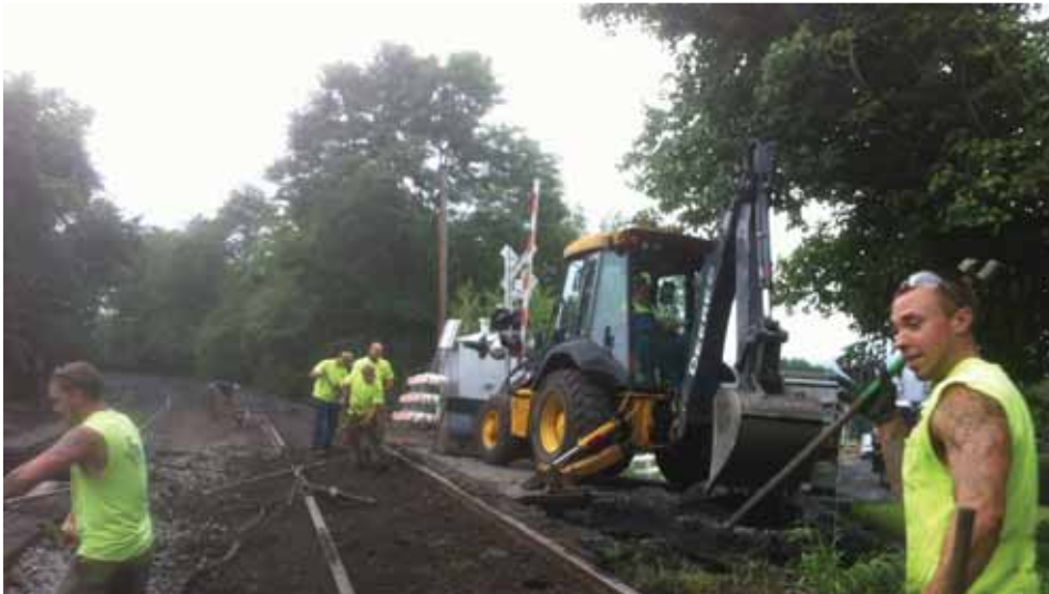
MOW forces beginning to dig up the old asphalt and a dirty ballast through the Broad Street crossing on #2 track MP 174.56. Left to Right: Nick Albertswerth, Matt Nester, Vince McGuigan, and Matt Minnich.
