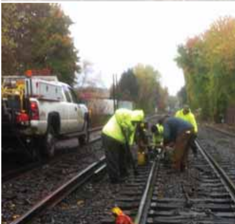
MOW forces connecting the rail on #2 track to make room for the new #20 switch that will be adding into Dupont Interlocking MP 175.5.
