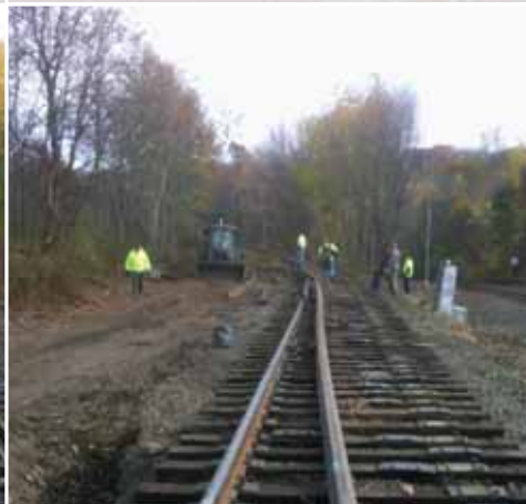
Grading, realigning, and changing rail on the CP connecting track at Dupont MP 175.5 to make the room needed to add two #20 equilateral switches into the interlocking.
