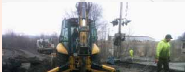
Track 1 has the rail removed and in the process of getting the ties out as crossing replacement is in full swing at Oak Street MP 173.13.
