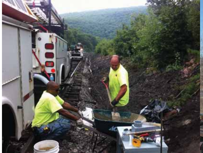
Maintainers Matt Collins and Darnell Young mix concrete to build a power transformer pad to supply high voltage power to the interlocking, nearly 2000' away.
