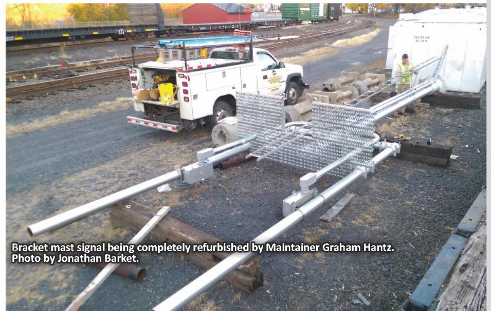
Signal heads being installed on bracket mast. Maintainer Dave Hutton giving directions to operator Matt Collins. Photo by Jonathan Barket.
