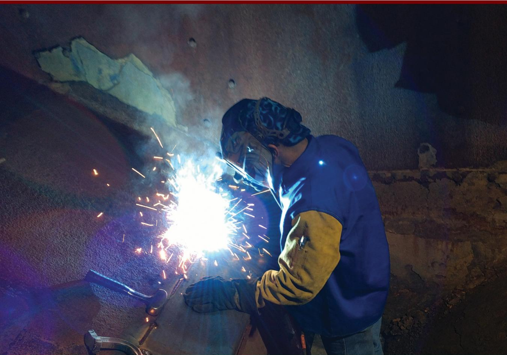
John Dubick performing repairs on the inside of one of our open top coal cars.
