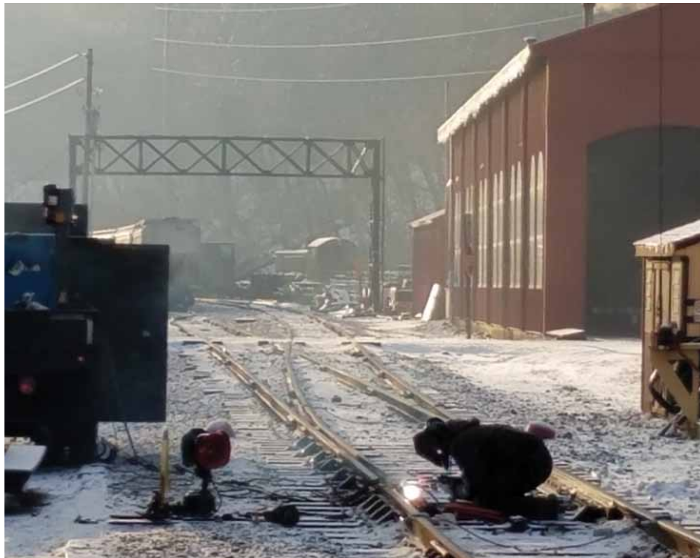
Aaron Cassel makes repairs to the switch point at the north end of Pulpit Rock siding, in Port Clinton. Photo by Daren Geschwindt.
