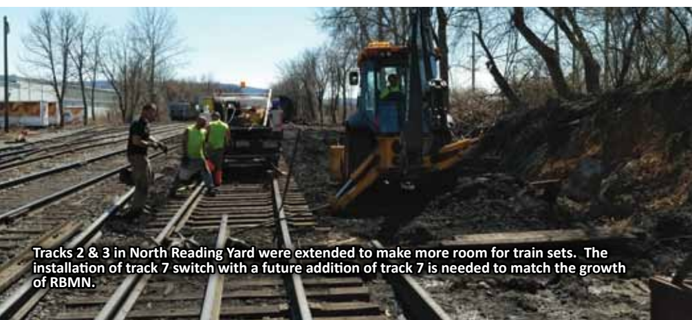
Shawn Himmelberger (backhoe) with Justin Hughes, Brandon Wagner, Jason Shupp, Matt Minnich, and Ben Cole are replacing timbers in Middle Yard switch MP 97.5. In the back of the picture is Dale Homm (backhoe) with Matt Sloskey working on the 2/3 switch.
