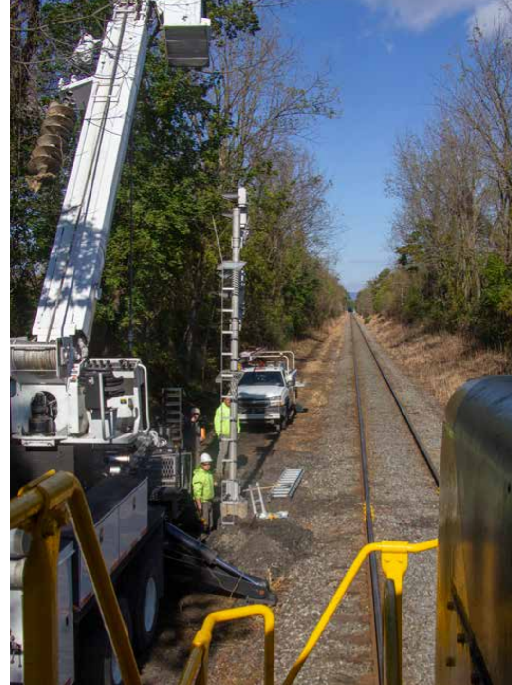
The North Reading Fast Freight eases past a crew installing CTC signals at Leesport, Pa., on Oct. 25, 2018. The railroad plans to have CTC operating over the length of its Main Line this year.
