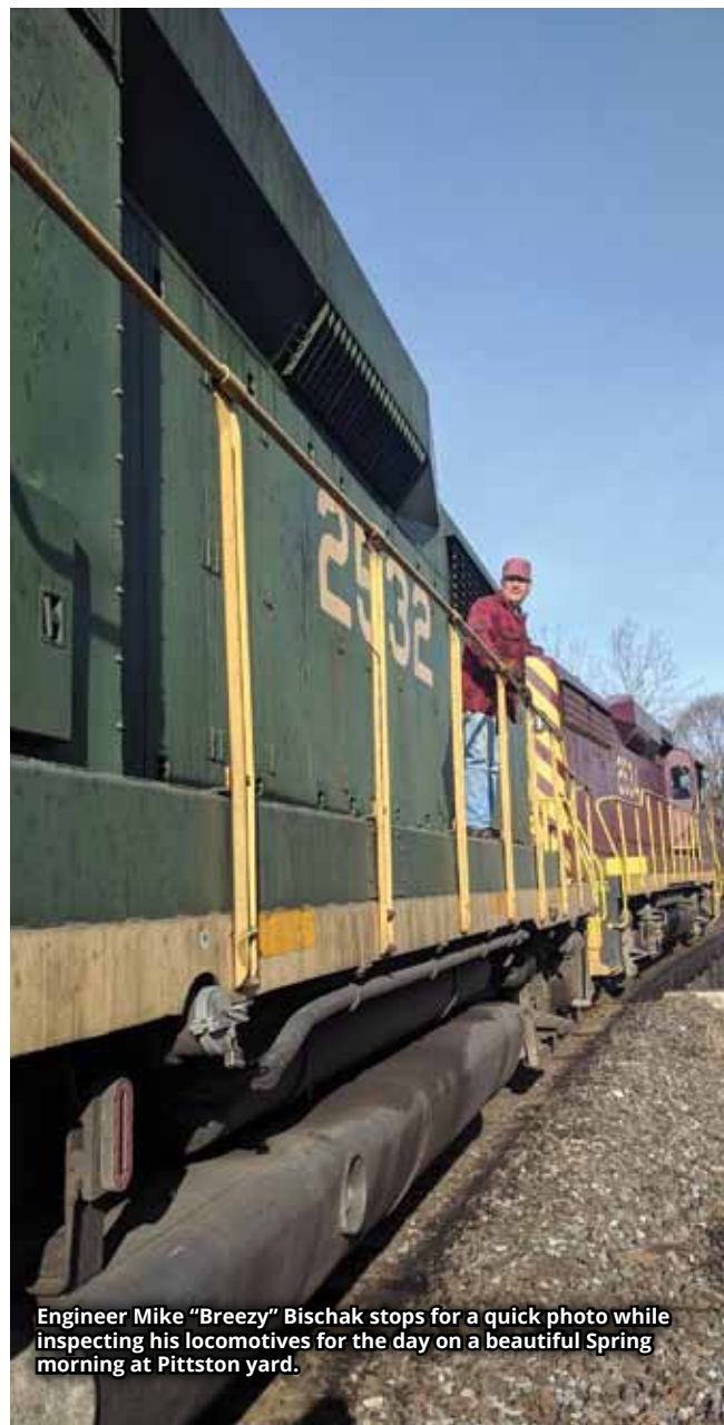
Ryan Bausher and Chuck Trusdell work underneath the boiler of steam locomotive 2102.
