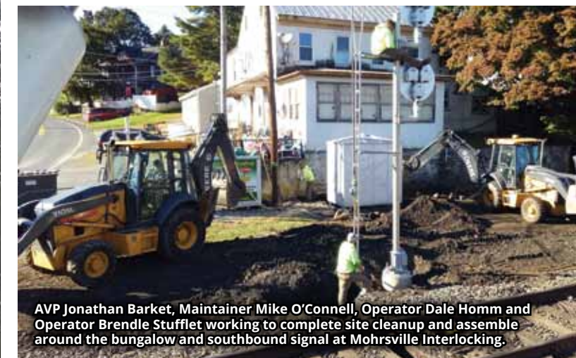
AVP Jonathan Barket, Maintainers Mike O'Connell, Graham Hantz, and Operator Brendle Stufflet working opening ground for cables to installed as part of the Mohrsville Interlocking Project.
