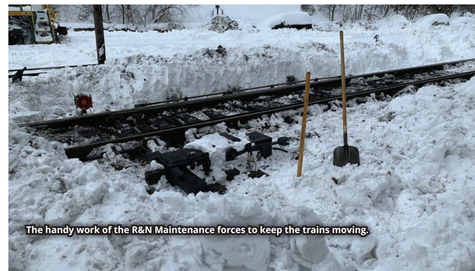
The Snow Warrior, WHHB2 Conductor Tom Skrutski, cleaning out switches to spot cars at PFN
