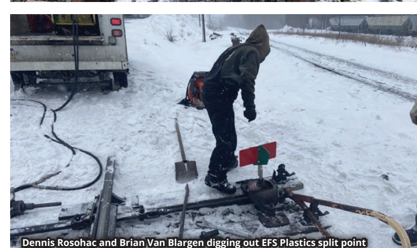
Dennis Rosohac and Brian Van Blargen digging out EFS Plastics split point derail.
