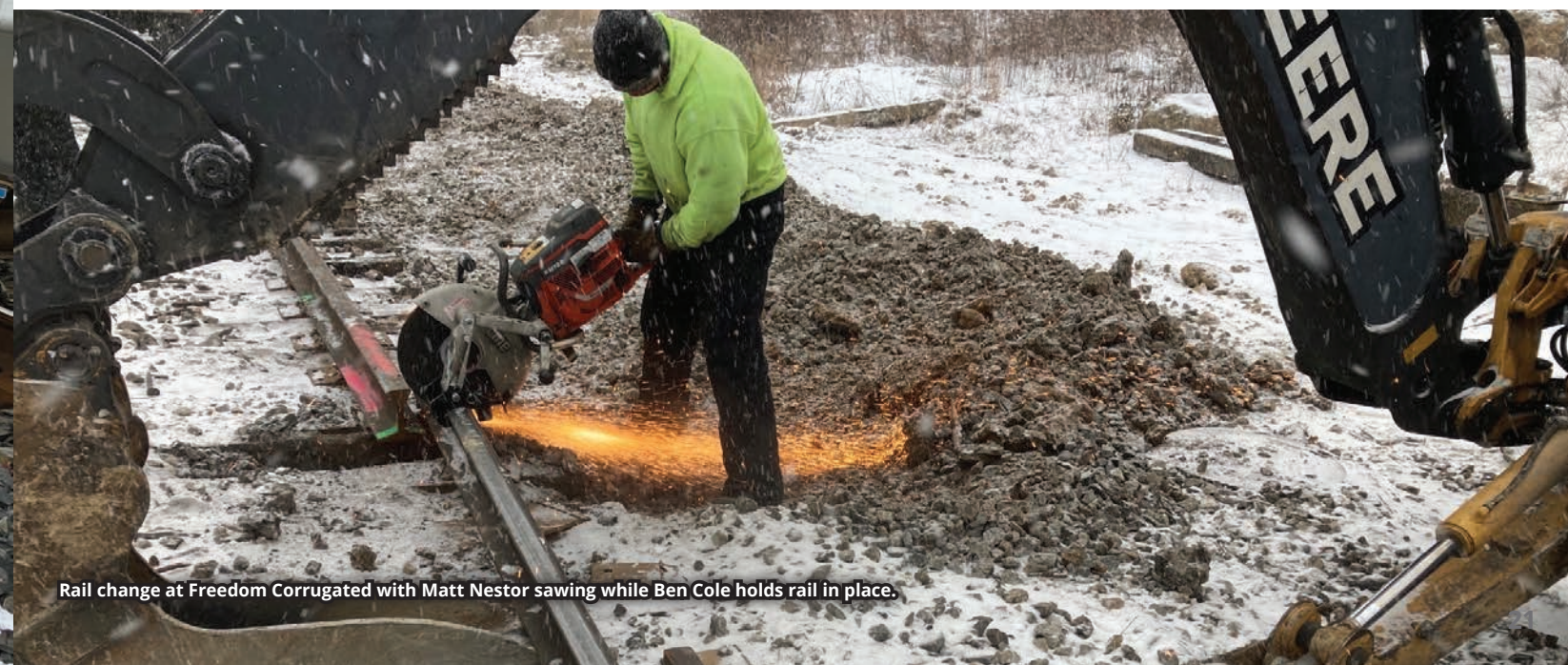
Chris Garcia, Josh Antosh, Matt McGinnis & Ben Cole in backhoe replacing rail Freedom Corrugated.
